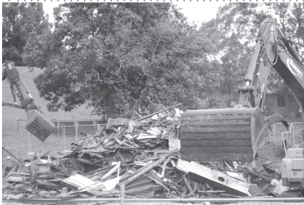
(Left) The clean-up of the pub ruins in progress. Photo by Paul Stobbie
