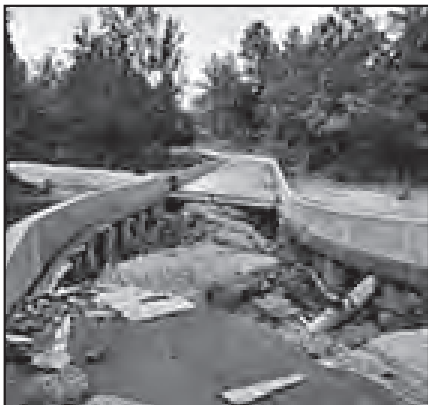
Tweed River Bridge after the March 2022 flood
